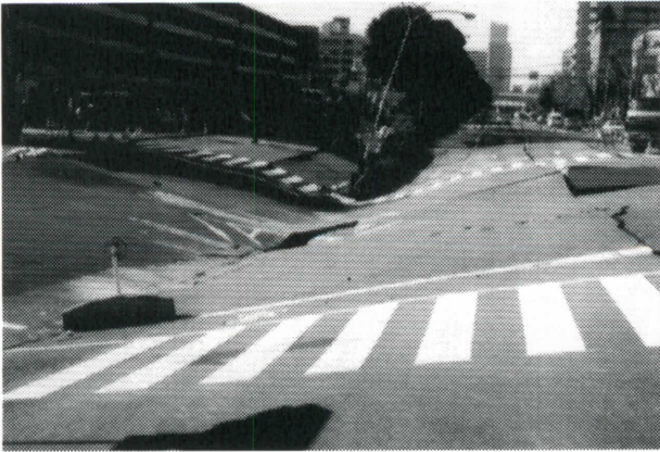
Photo.1 Subsidence of the pavement occurred over the subway station
