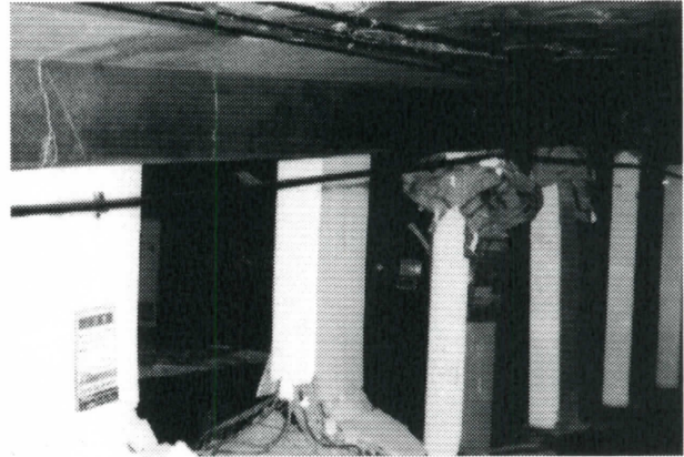
Photo.4 Buckling of center columns (the third pattern of collapse)
